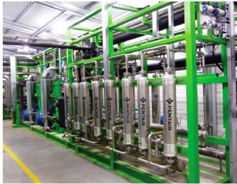
Figure 2: gas upgrading membranes at the Wijster green gas hub
